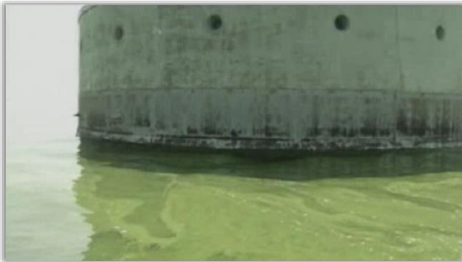
Water Intake, Water line courtesy – ClickOn Detroit
