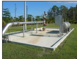
Deep injection well
