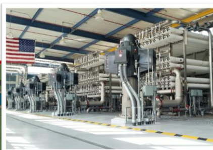
Kay Bailey Hutchison Brackish Groundwater Desalination Plant, TX
