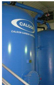
Granular Activated Carbon (GAC)
