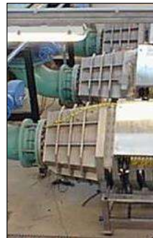
UV-Advanced Oxidation Process (UV-AOP)
