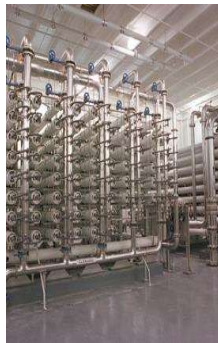
Low Pressure Reverse Osmosis (LPRO)
