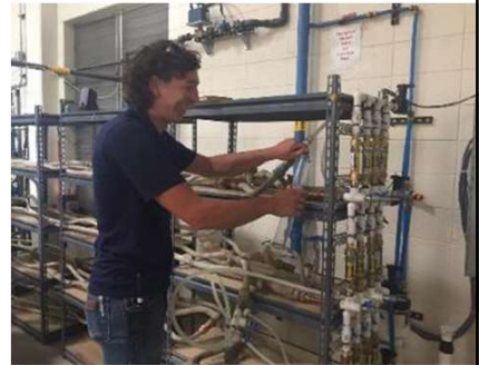
Marston's Lead Pipe Study, one of our two ongoing treatment pilots.
